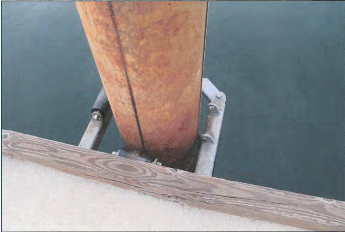
Figure 8. Missing Pile Bumpers
