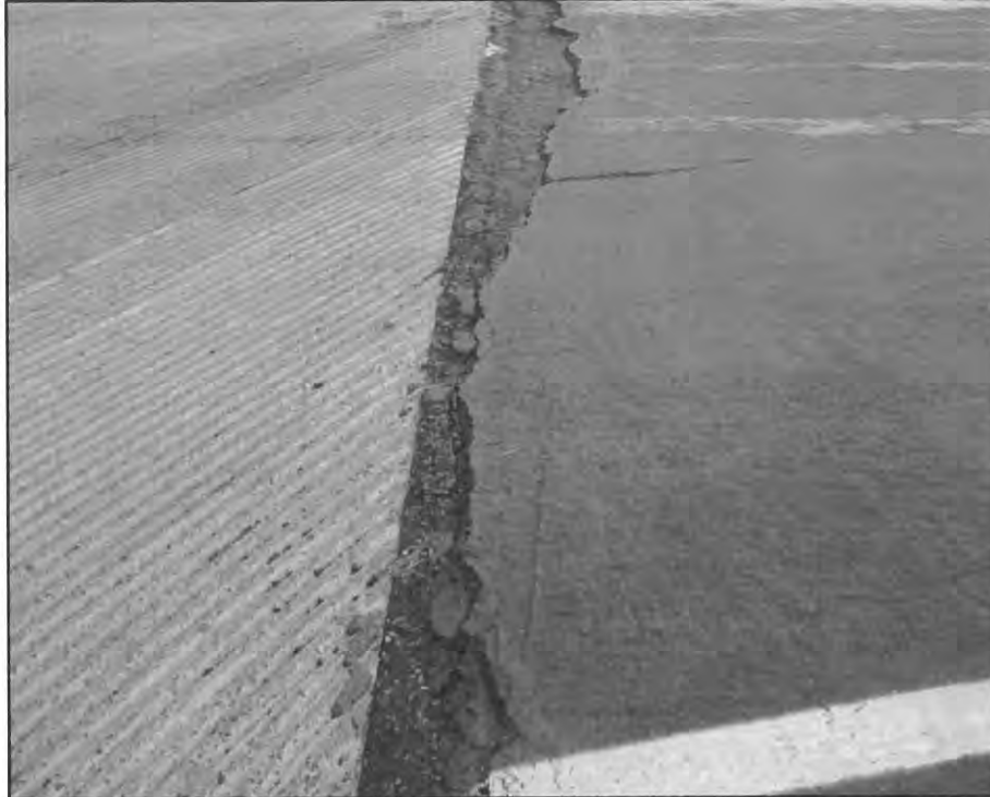
Figure 11. Asphalt chipping at Boat Launch Ramp
