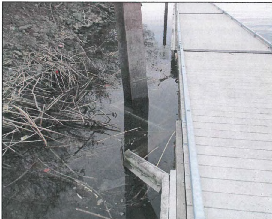
Figure 10. Damaged Dock Bumpers
